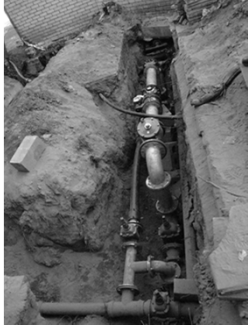
Standard Meter Installation
