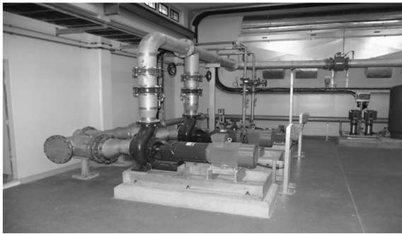
New machine room at Meulwater WTW
