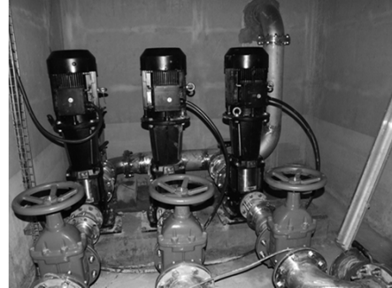
Upgraded Pump Station - Leliefontein Reservoir, Paarl
